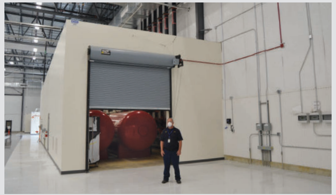
Foam equipment room shown here was constructed to house main and reserve foam tanks, system risers, fire pumps and controls.
