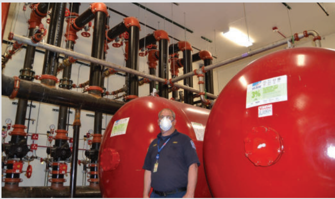
Multiple foam-water deluge systems protecting the entire hangar floor space. Each deluge system protected an area over 9,000 square feet each.
