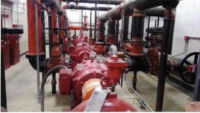
Four 2,500 gpm electric fire pumps were installed and supplied by a new 16" ductile feed into the building.
