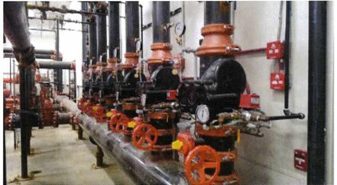
Foam-water deluge systems protecting the entire hangar floor space. Each deluge system protected an area over 9,000 square feet each.
