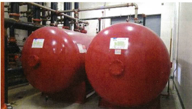
Two 2,600-gallon bladder tanks containing a total of 5,200 gallons of RE-HEALING 3% Fluorine-free foam.
